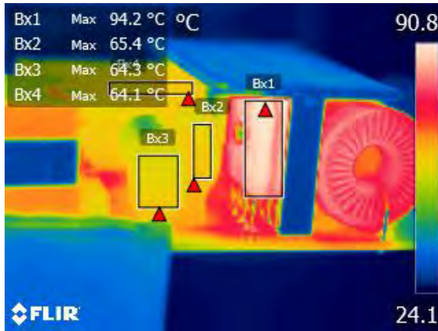
Figure 64– Bridge Rectifier Side Thermal Picture, 100% Load, 90 VAC.
