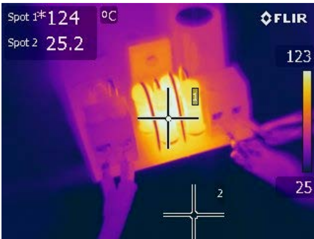
Figure 42 – 115 V VAC, 30 V LED Load, 0 V dim. Spot 1: Pre-Load Resistors (R51-60): 124 °C.
