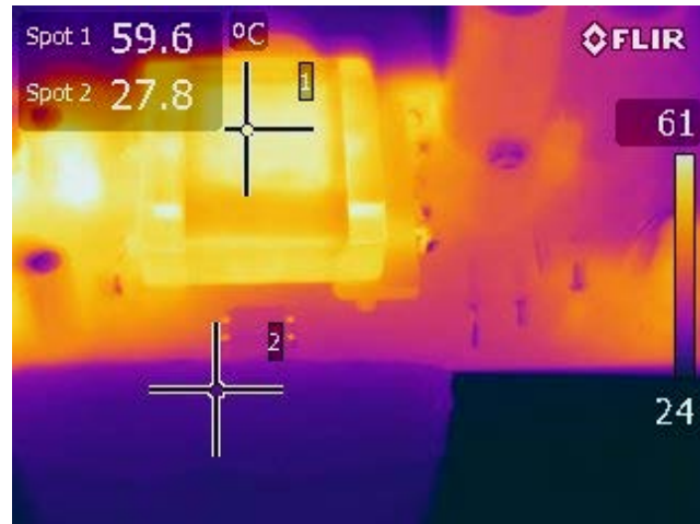
Figure 26 – 132 V VAC, Full Load. Spot 1: Transformer (T1): 59.6 °C.
