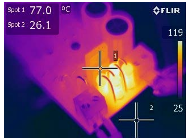
Figure 43 – 115 V VAC, 30 V LED Load, 0 V Dim. Spot 1: Pre-Load Switch (Q6): 77 °C.
